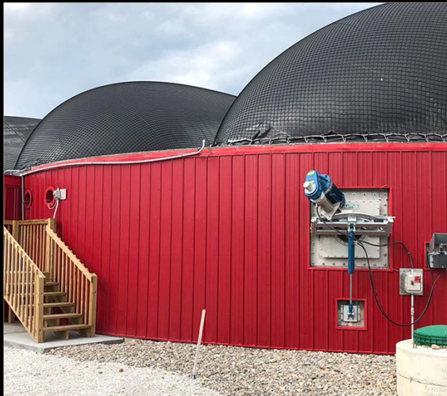
Dairy Farm Biogas Facility
